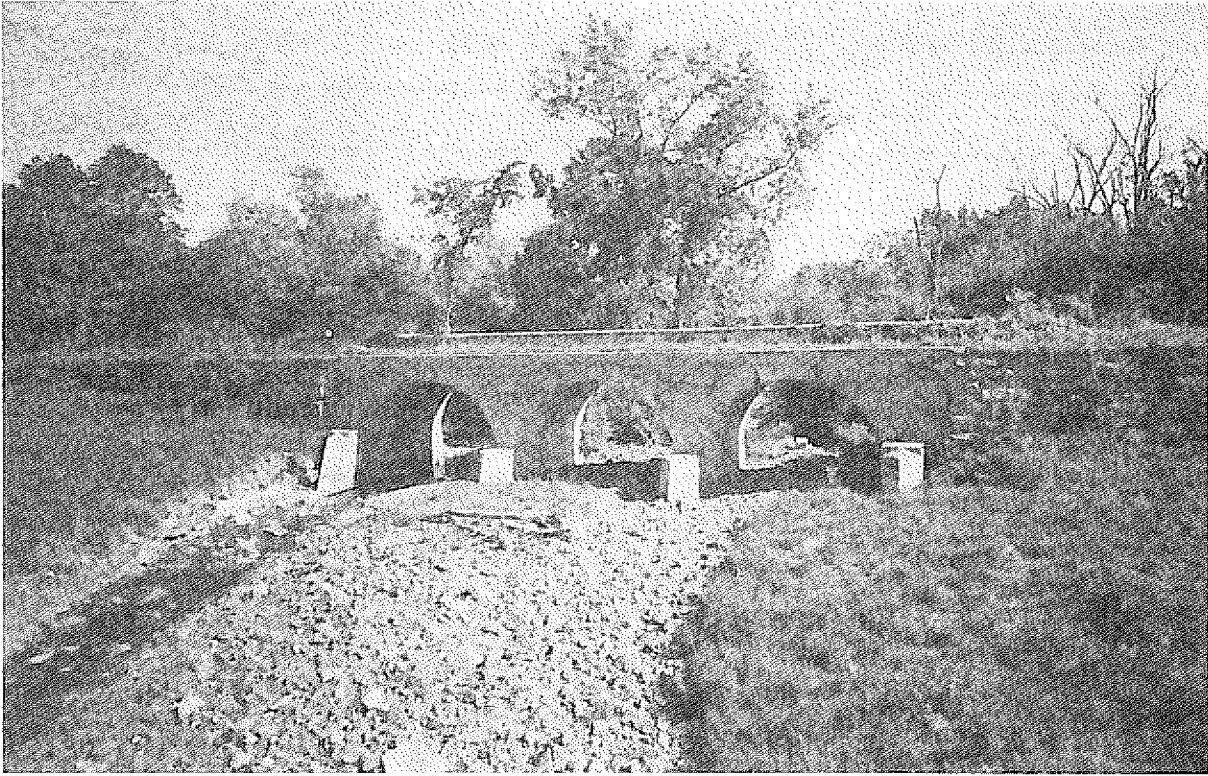
FIGURE 12 Early Erie Canal stone masonry towpath bridge near Rotterdam, New York, now part of an improved bicycle path. (Photo from New York State Office of Parks, Recreation and Historic Preservation.)
